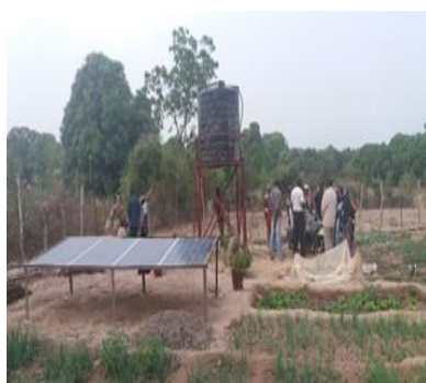
Solar pump at Garalo site
